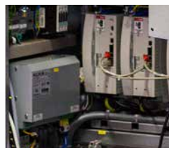
Controllers, inverters/ servo amplifiers & power packs
